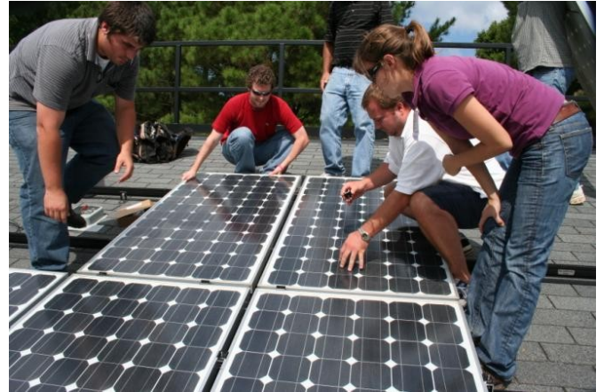
The Solar Center provides training programs and equipment to North Carolina's industry professionals and renewable energy firms.
