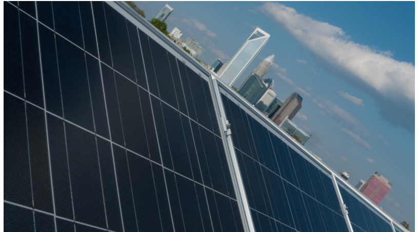
Photo courtesy of Argand Energy
